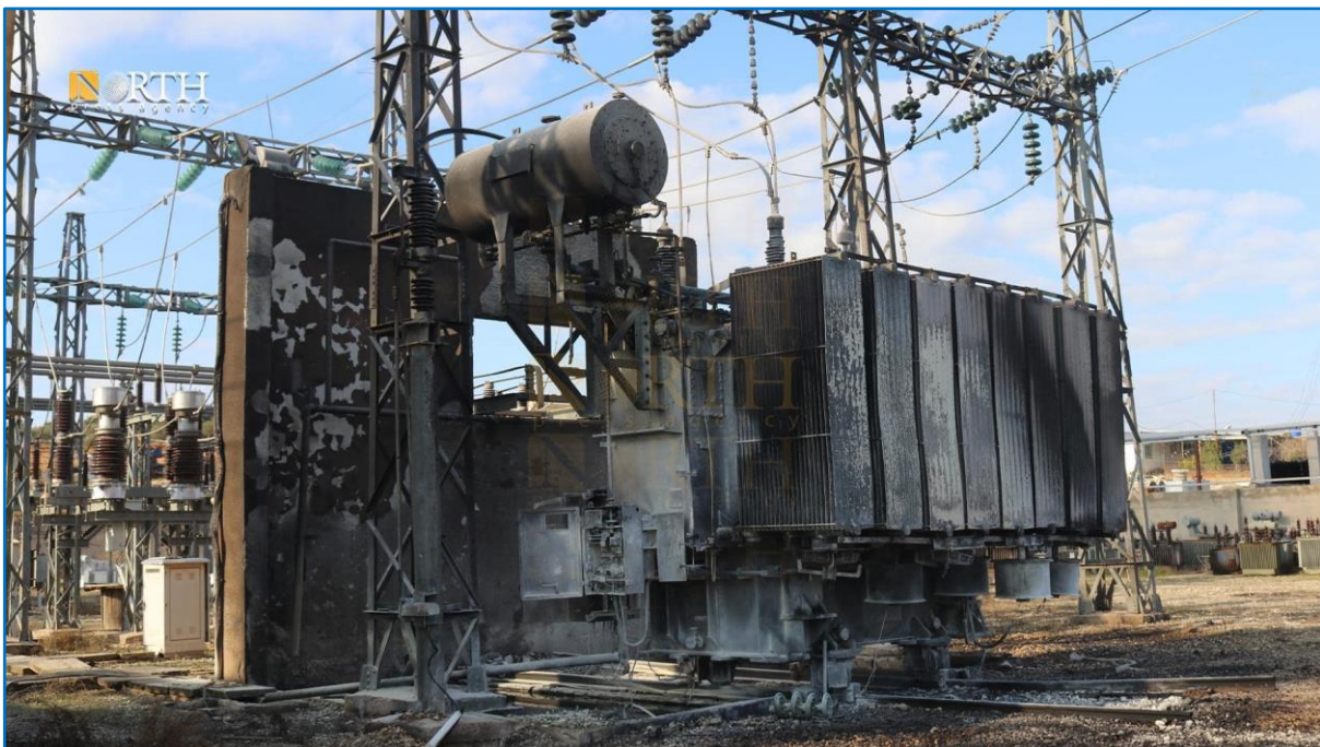
Images showing fires in a power transfer station in Kobani City after it was hit by a Turkish drone in mid-January 2024. Photos Source: North Press Agency
