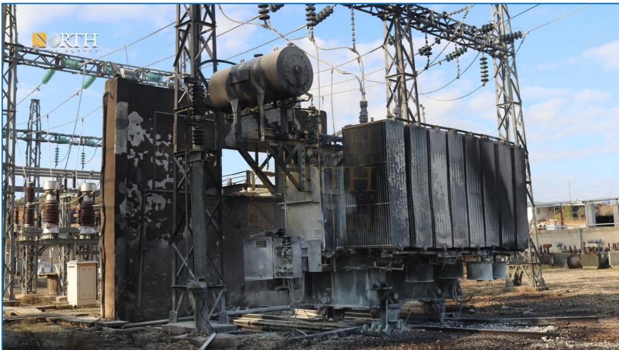
Images showing fires in a power transfer station in Kobani City after it was targeted by a Turkish drone in mid-January 2024. Photos Source: North Press Agency
