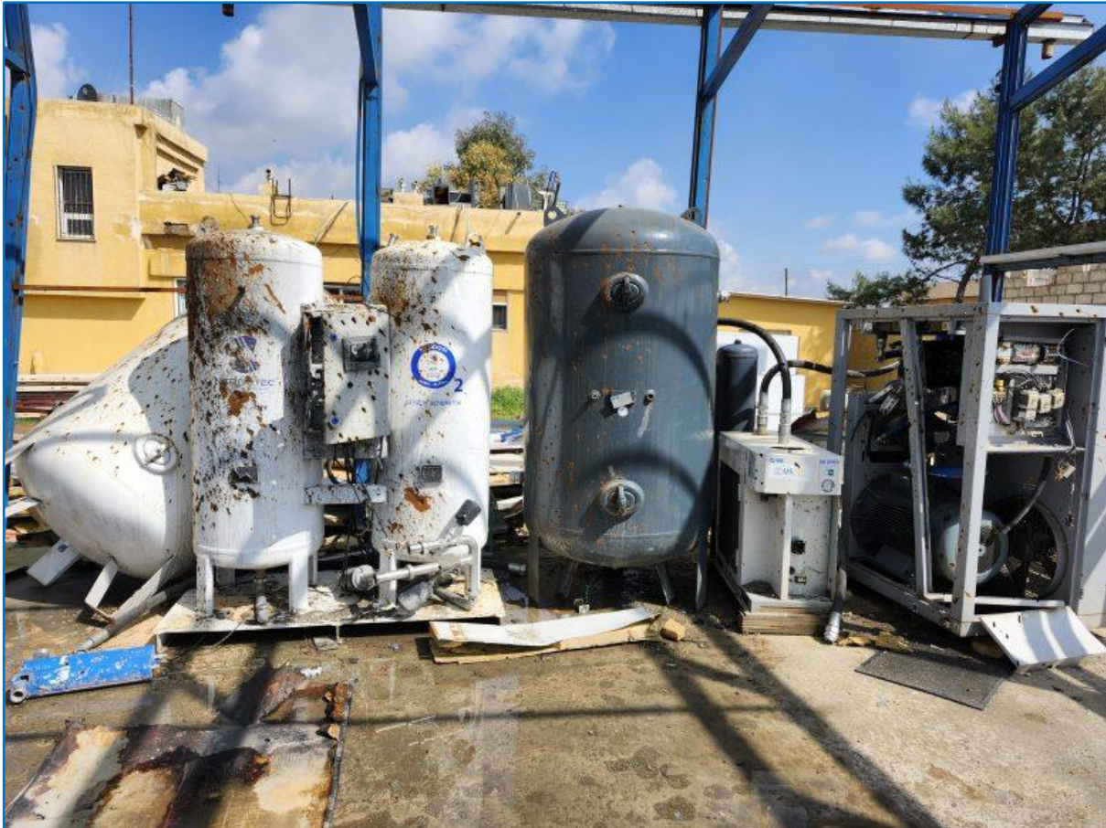
An image of the destroyed Qamishli-based oxygen bottling plant, taken on March 10, 2024, by Meghan Bodette , Director of Research at the Kurdish Peace Institute (KPI). The photo was published in a report titled “Turkey Targets USAID Projects in Northeast Syria”. Photo Source: KPI
