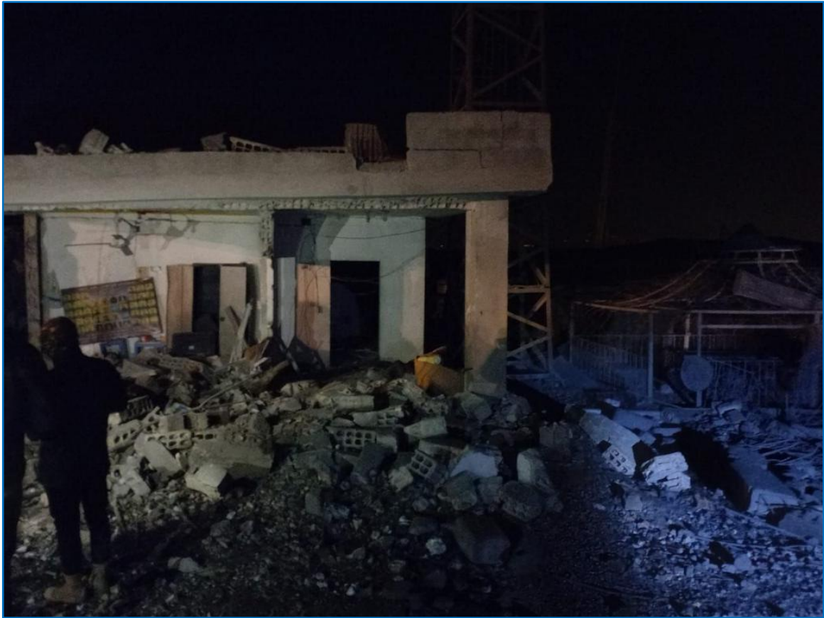
An image showing aftermath of the Turkish two consecutive drones attacks on the power plant in Taql Baql Village in al-Malikiyah/Derik countryside on November 20, 2022. Photo Credit: Hawar News Agency.
